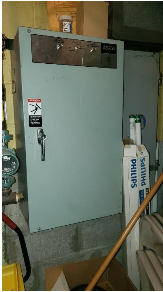
Photograph 2 – Existing Automatic Transfer Switch in Building
