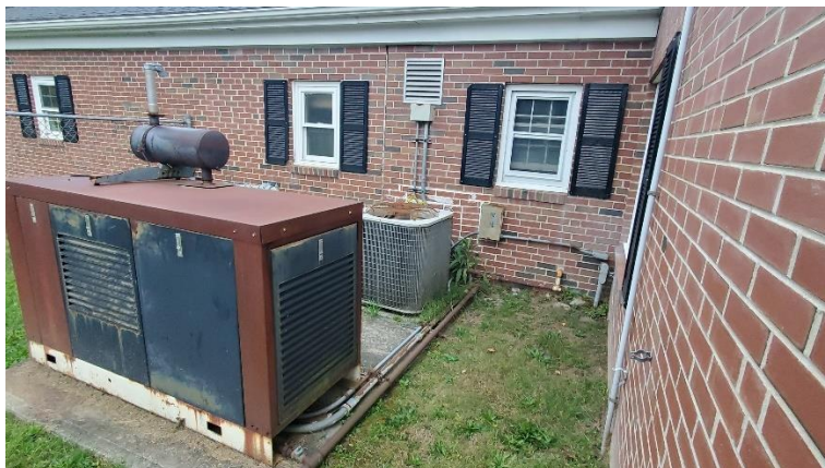
Photograph 1 – Existing 30KVA Generator Outside of Building
